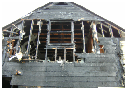
A recent fire destroyed this home..
